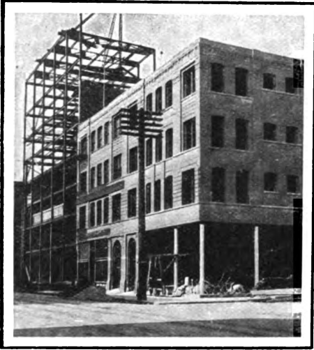
TWO BUILDINGS IN COURSE OF CONSTRUCTION ON FIFTH STREET, PORTLAND—THE NEW RETAIL DISTRICT. THE STEEL STRUCTURE IS THAT OF THE COMMERCIAL CLUB. ALL PHOTOGRAPHS SHOWING BUILDINGS IN COURSE OF CONSTRUCTION, AND USED TO ILLUSTRATE THIS ARTICLE, WERE TAKEN THE SAME WEEK, SHOWING AS REMARKABLE BUILDING PROGRESS AS ANY IN THE UNITED STATES. THE INCREASE IN BUILDING IN APRIL, 1907, OVER 1906, WAS 167 PER CENT, SO THAT PRACTICALLY A NEW CITY IS BEING ERRECTED IN PORTLAND TO-DAY
